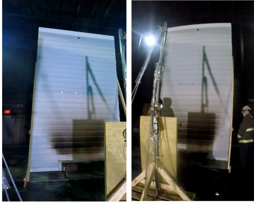
Figure 25 - Post-test Photographs of Test 7 Fiber Cement Siding/EPS/Mineral Wool Wall Assembly with 75 kW Ignition Prior to Panel Removal
